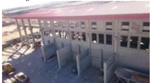
Figure 15: the concrete structure warehouse. The fourth case is Concrete that has 2000m 2 area (65*30.7). After knowing the quantity of concrete in this case study which is 1449 m 3 , when the density of the concrete is 2400kg/m 3 .
